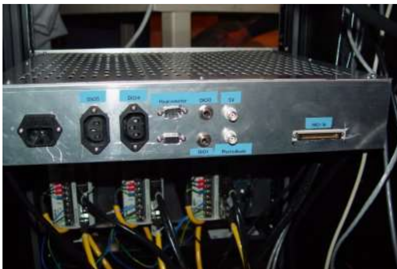
Figure 8. View of the rear of the rack-mount enclosure housing the predecessor of the 1901 board. From the left: one 120VAC receptacle, two 120VAC sockets, hygrometer “D” connector, Unused “D” connector, gas solenoid power jacks, 5VDC supply for the droplet detector laser, 5VDC BNC for the the droplet detector photodiode, and 68-pin interface board connector.
